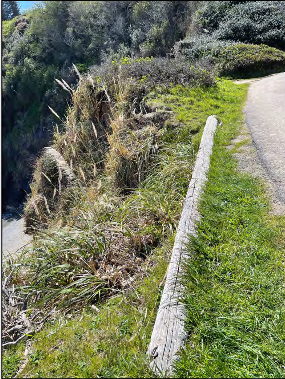
Figure 28. Coastal Erosion Encroaching on the Trinidad Head Access Road.
