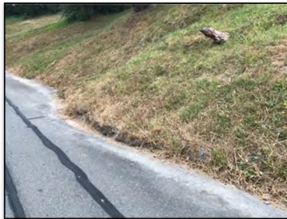
Figure 32. Erosion/slide on Cher-Ae Lane.
