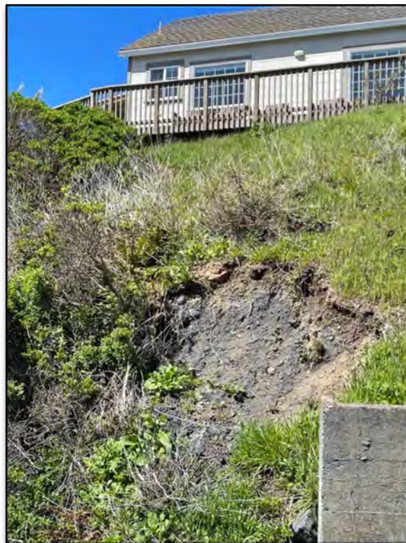
Figure 30. Erosion Below Seascapes House (Trinidad Head Access Road to left).
