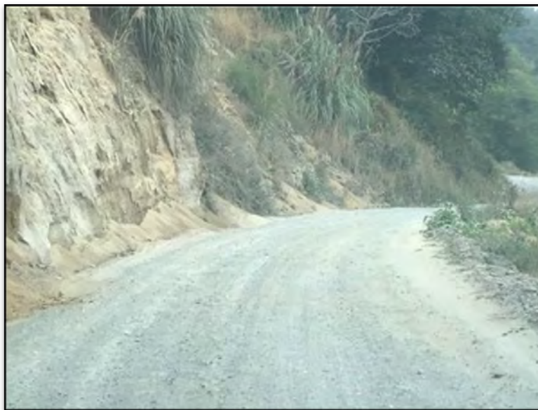
Figure 35. Scenic Drive Pavement Erosion.
