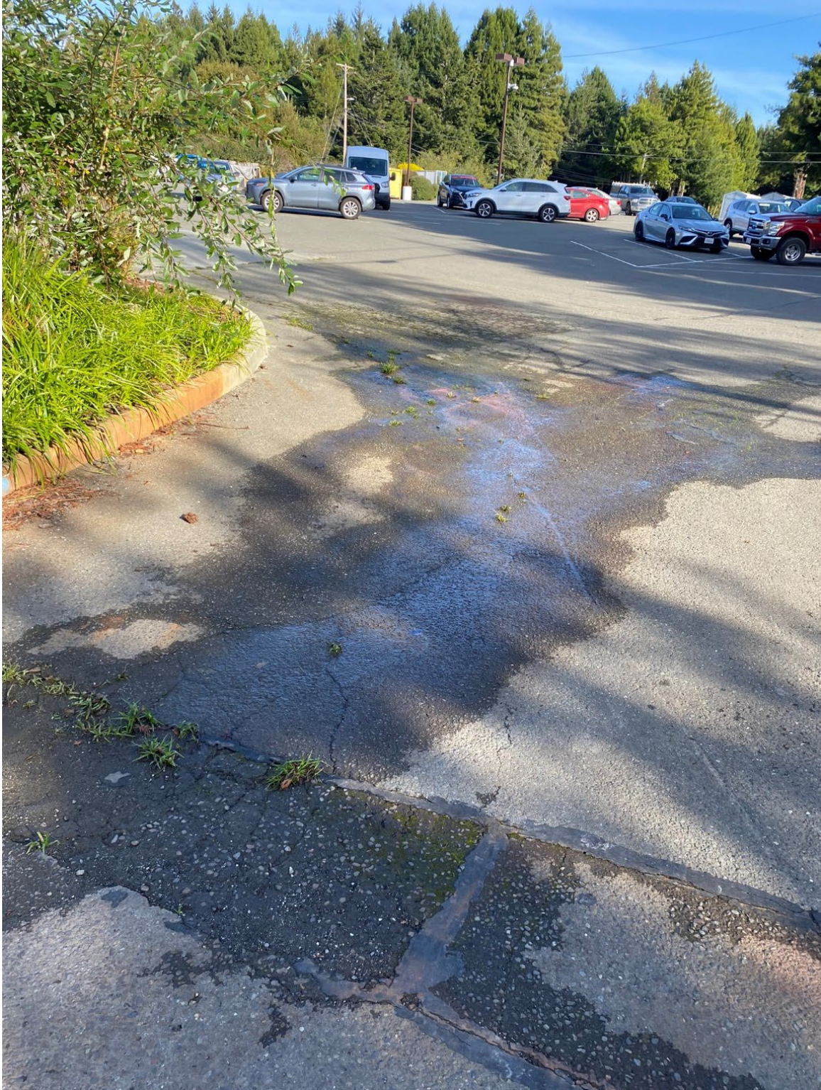
Figure 5: Contributing Drainage Area South of Inlet, Water surfacing from hydrostatic pressure, North side of Ma-We-Mor View Ln
